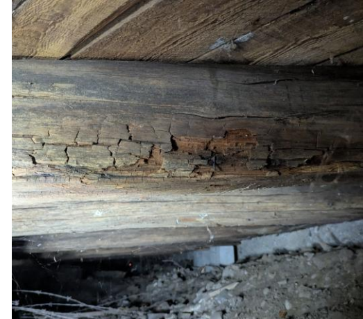
FIGURE 10: Timber Beam Rot
