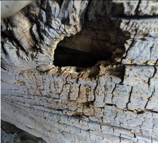
FIGURE 7: Very Severe Rot
