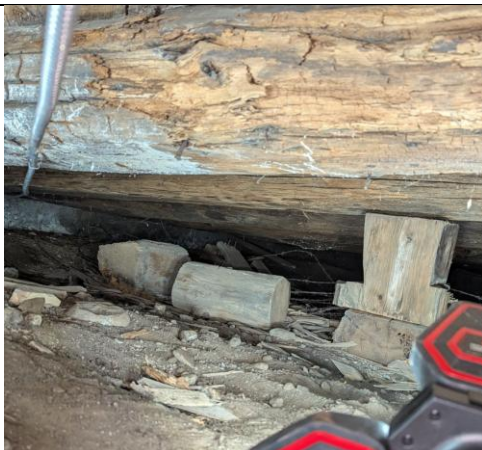
FIGURE 11: Makeshift Timber Post
