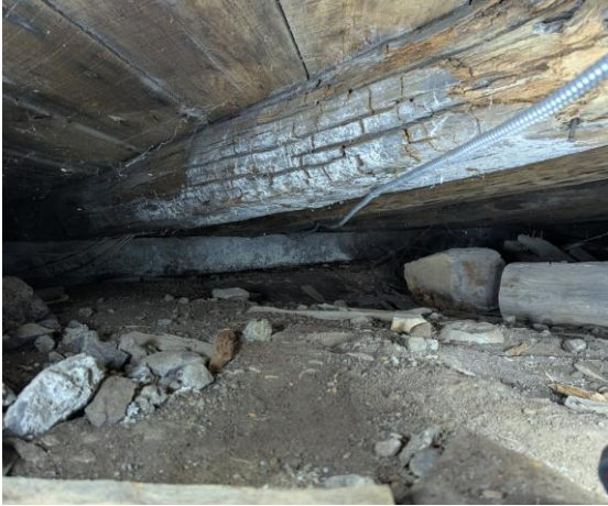
FIGURE 9: Timber Beam Rot
