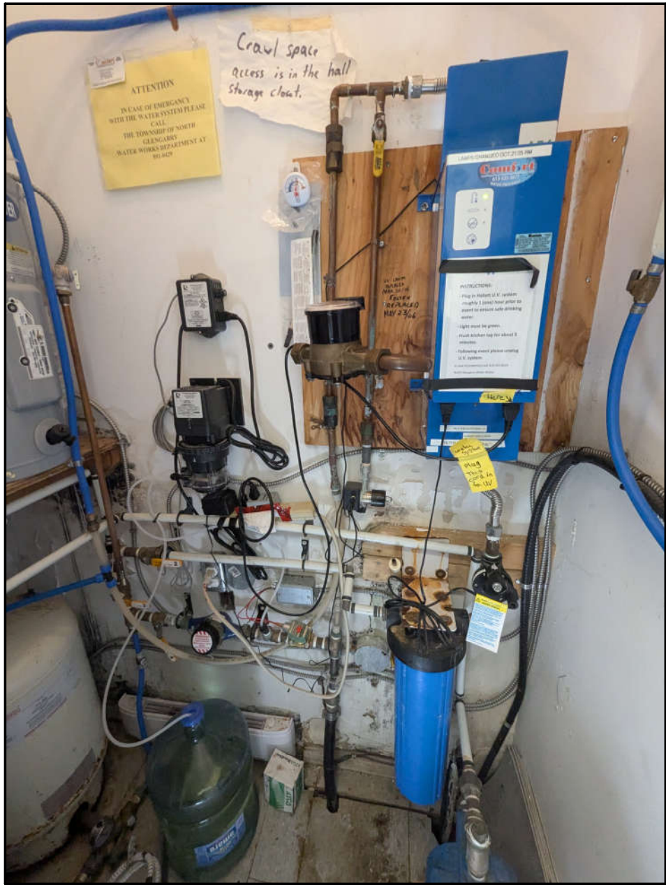
PHOTO - EXISTING MECHANICAL ROOM
