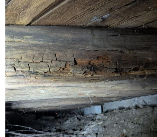
FIGURE 10: Timber Beam Rot
