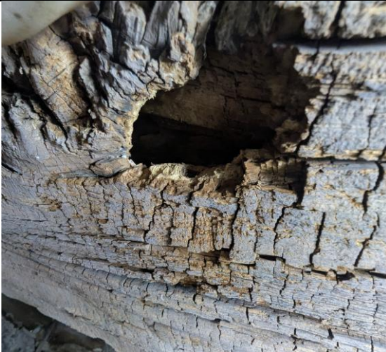
FIGURE 7: Very Severe Rot
